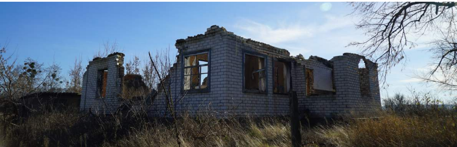
Damaged house in Bohorodychne village, Donetsk region
