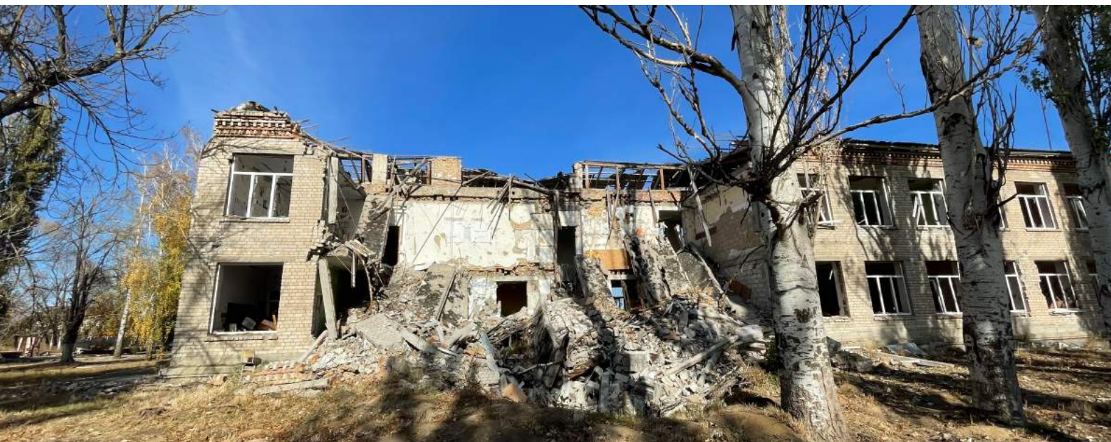
Destroyed school in Pervomaiske settlement, Mykolaiv region
